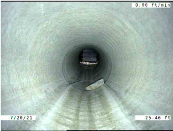
CB010016-CB01016A_8af9cc66-3db8-4760-8e84-a8409a051a45_20210720_180652_406.jpg, 00:04:05, 25.46ft Crack Multiple from 4 o'clock to 12 o'clock, within 8 inch, Finish
