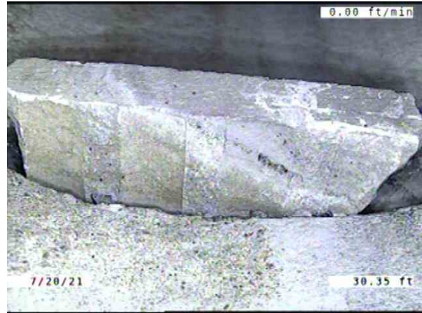
CB010016-CB01016A_060db97e-219d-450f-9333-9e583b1b32df_20210720_180749_288.jpg, 00:04:36, 30.35ft Obstruction Wedged In The Joint, 10% of cross sectional area from 4 o'clock to 6 o'clock, within 8 inch / LOOKS LIKE A PIECE OF TILE
