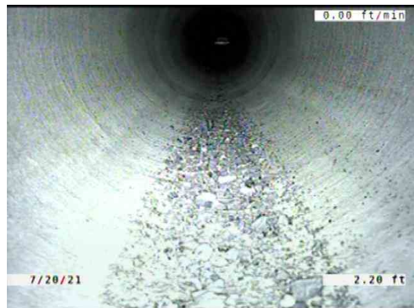
CB010016-CB01016A_edb52a8a-8cc7-4f19-a29d-e89346bb57f3_20210720_175649_226.jpg, 00:00:39, 2.20ft Deposits Settled Fine, 5% of cross sectional area from 5 o'clock to 7 o'clock, within 8 inch, Start
