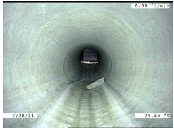
CB010016-CB01016A_b5863c2f-b0e4-4595-a674-2fb0ae384d43_20210720_180628_792.jpg, 00:03:56, 25.45ft Deposits Settled Fine, 5% of cross sectional area from 5 o'clock to 7 o'clock, within 8 inch, Finish
