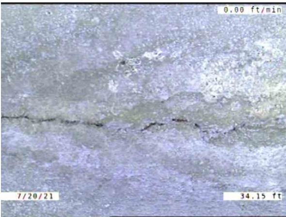
CB010016-CB01016A_b0af1ef9-d983-4076-a33f-e91eb4c8ed24_20210720_180856_841.jpg, 00:05:34, 34.15ft Crack Circumferential from 12 o'clock to 12 o'clock
