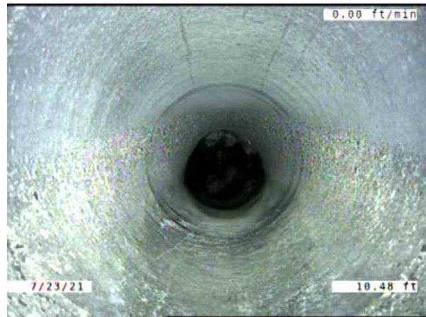
CB010025-CB01065B_c53109af-2e1b-470e-9483-cb1390b7a348_20210723_125949_214.jpg, 00:03:19, 10.48ft Surface Damage Aggregate Visible from 12 o'clock to 12 o'clock, within 8 inch, Start
