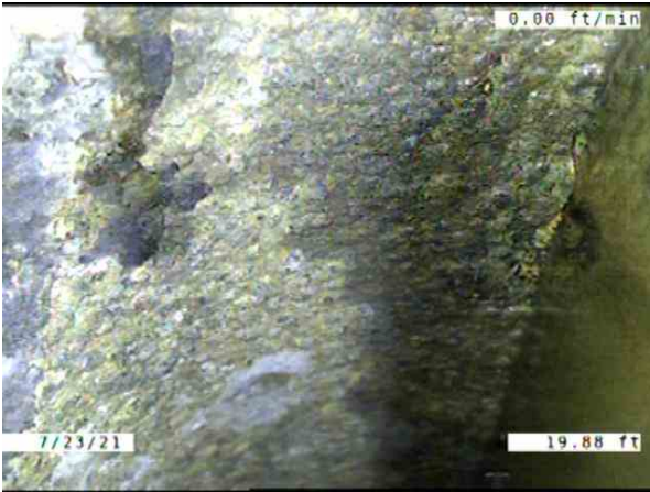
CB010025-CB01065B_851a551f-b992-4e5d-96b6-e7666cfb1002_20210723_130630_248.jpg, 00:08:03, 19.88ft Surface Spalling of Damage Coating from 9 o'clock to 3 o'clock, within 8 inch
