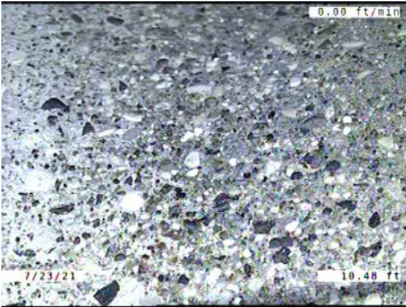
CB010025-CB01065B_67719e4b-8ec2-45bd-a992-b97a42db27c2_20210723_125956_295.jpg, 00:03:19, 10.48ft Surface Damage Aggregate Visible from 12 o'clock to 12 o'clock, within 8 inch, Start
