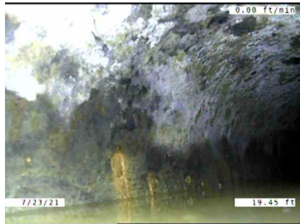
CB010025-CB01065B_719ae133-4872-43aa-9934-81379db87ee9_20210723_130403_108.jpg, 00:06:34, 19.45ft Surface Damage Aggregate Visible from 12 o'clock to 12 o'clock, within 8 inch, Finish
