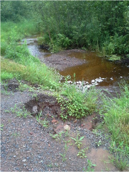
#3 West end of Blueberry Rd
