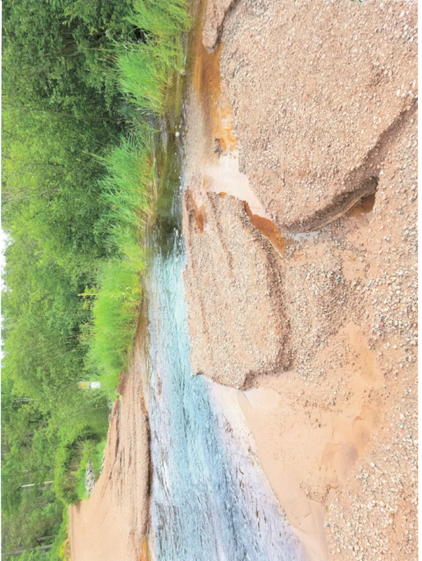
#Smiles Lake Rd Culverts. Water washed out the Road
