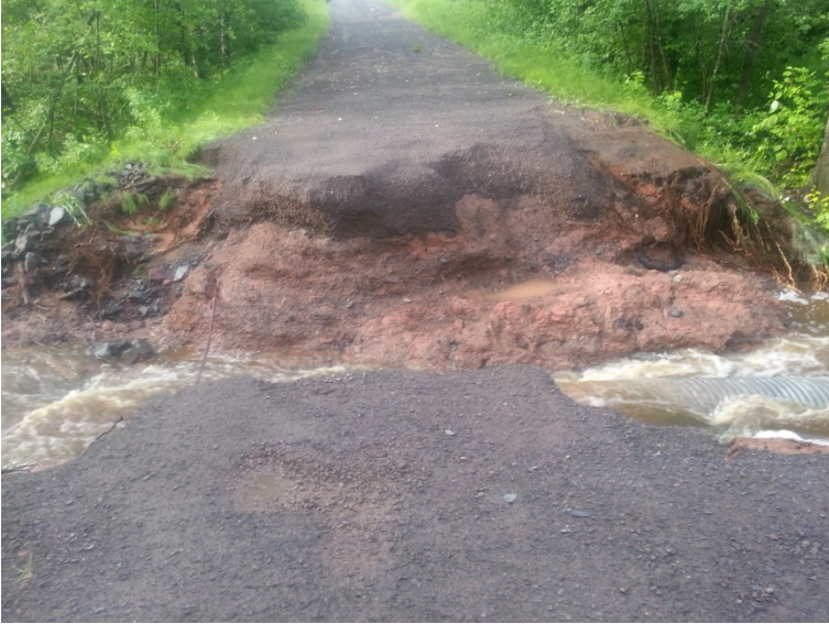
#1 Logan Ave. looking South (Damaged Culvert)
