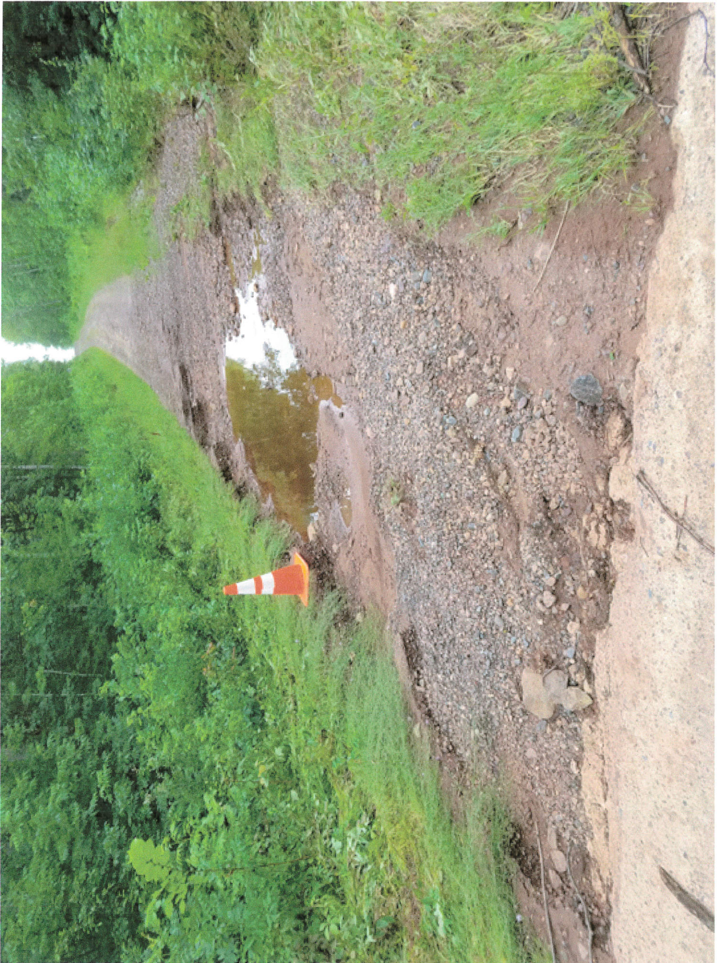
#1 Bridge on Crotte Brook Rd East side of Bridge washed out
