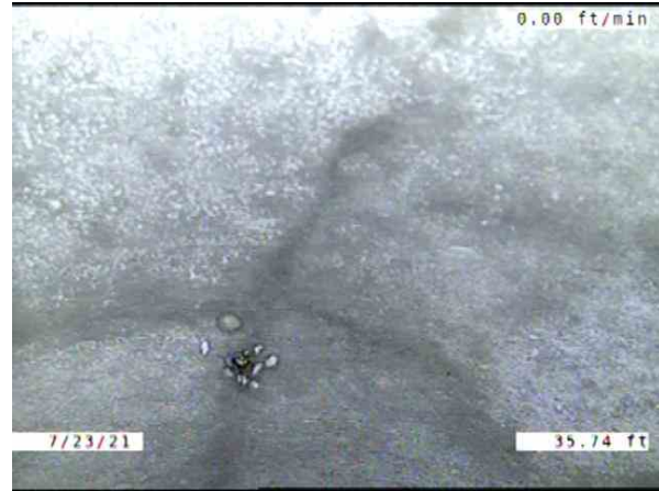
CB01001B-CB01001C_aa0a4938-e6d5-4f09-bb8d-a2ffdb32948e_20210723_164324_298.jpg, 00:06:50, 35.74ft Crack Multiple from 10 o'clock to 5 o'clock, within 8 inch
