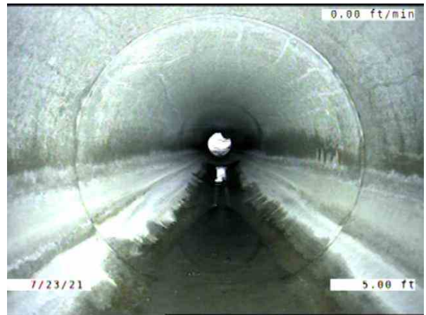
CB01001B-CB01001C_35ad9f59-5627-4e7c-ba6f-15be1e1ee5c9_20210723_163920_925.jpg, 00:03:03, 5.00ft Crack Multiple from 12 o'clock to 12 o'clock, within 8 inch, Finish
