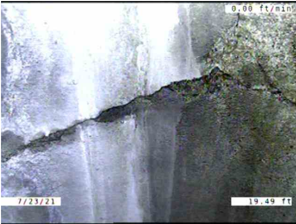
CB01001B-CB01001C_b21691ef-f58d-4c4a-8127-8b3cb49a4048_20210723_164124_797.jpg, 00:04:59, 19.49ft Broken from 12 o'clock to 11 o'clock, within 8 inch
