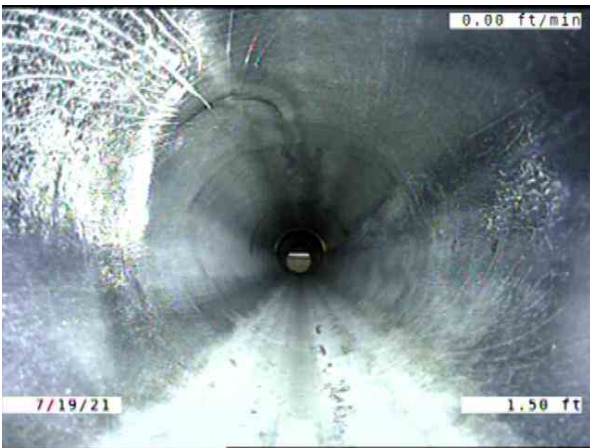
CB010024-CB010360_cfb3fe89-6bf9-4ea6-8d8c-f9bad42dd560_20210719_155944_433.jpg, 00:00:18, 1.50ft Miscellaneous General Observation / DROP INTO THE CATCH BASIN. HAD TO START IN THE PIPE.
