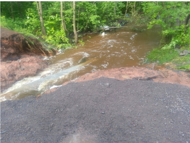
#1 Logan Ave Looking West (Damaged Culvert)
