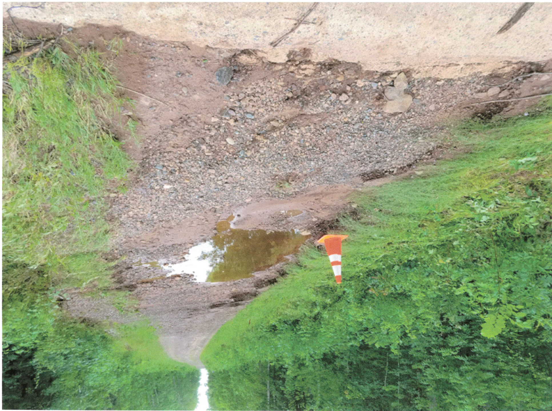
#1 Bridge on Crotte Brook Rd East side of Bridge washed out
