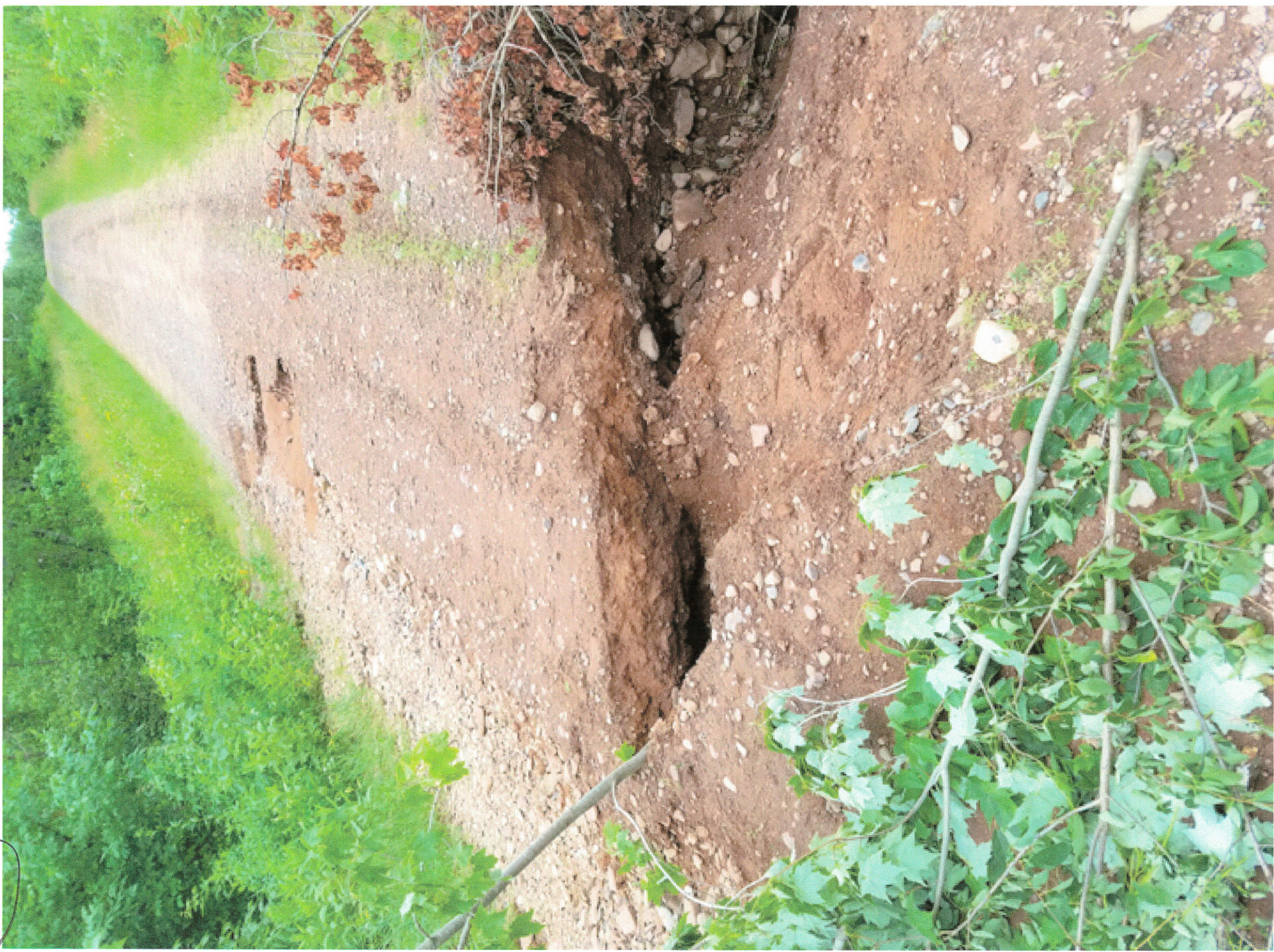
#2 Culverts on Crotte Brook Rd Washed out
