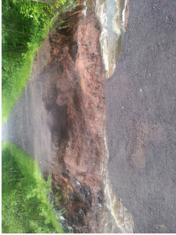
#1 Logan Ave. looking South (Damaged Culvert)
