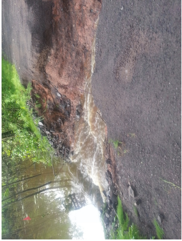
#1 Logan Ave. Looking East (DAMAGED CULVERT) Culvert was
