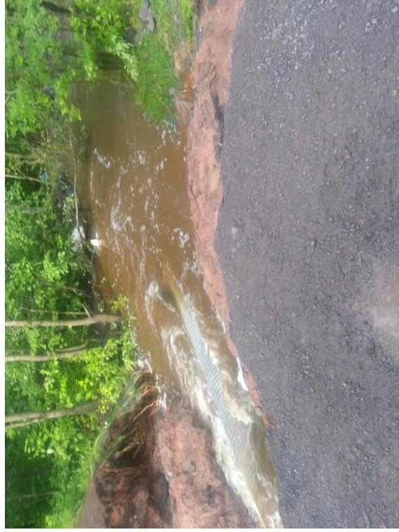
#1 Logan Ave Looking West (Damaged Culvert)
